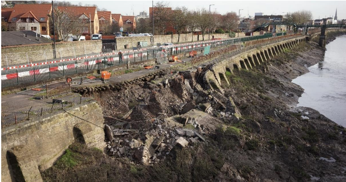
Figure 19 - Photo showing collapse of the riparian wall on Cumberland Road in 2019
