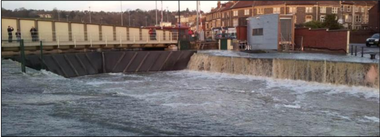
Figure 15 - Water shown overtopping the Junction Lock stop gates into the Floating Harbour
